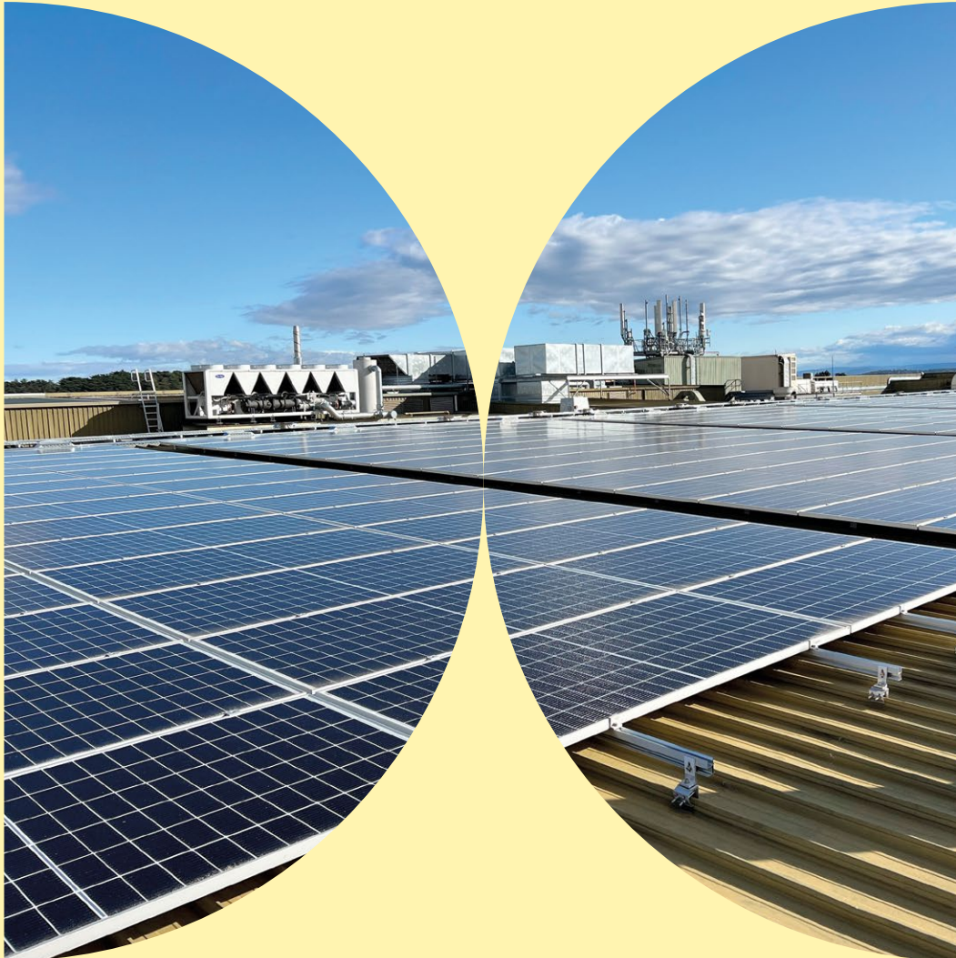
Chirnside Park, VIC, solar PV array
